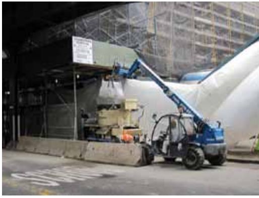
A self-contained machine was selected—one that far exceeded the necessary requirements for mixing volume and pumping distance and was capable of mixing bulk bags
