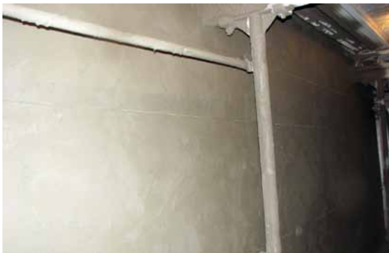
The uniformed float finish provided an excellent textured surface for the coating adhesion
