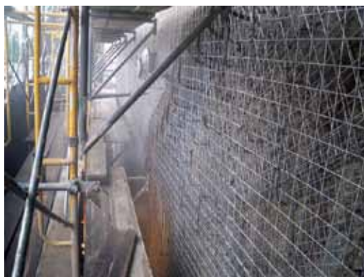
Double and triple mats of 4 x 4 in. (100 x 100 mm) welded-wire reinforcement installed in severely deteriorated locations
